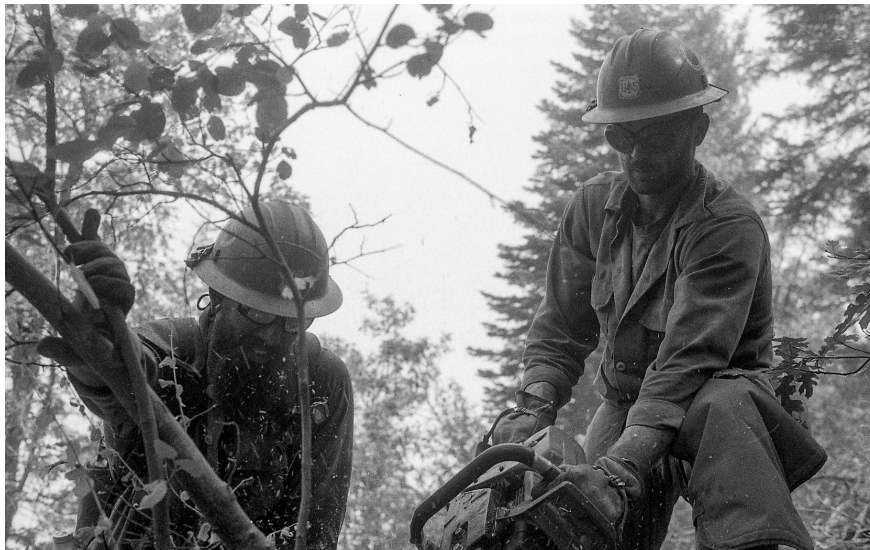
One of our saw teams cutting brush and removing it from the containment line. Image by: Evan Houston
